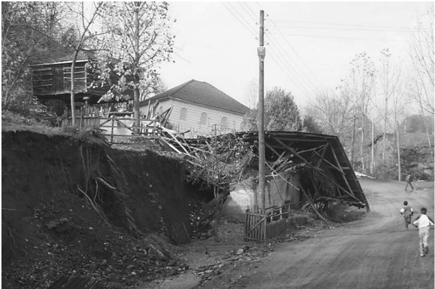
Fig. 4.5 Normal Fault in Turkey. Photo: R. Rothaus.
